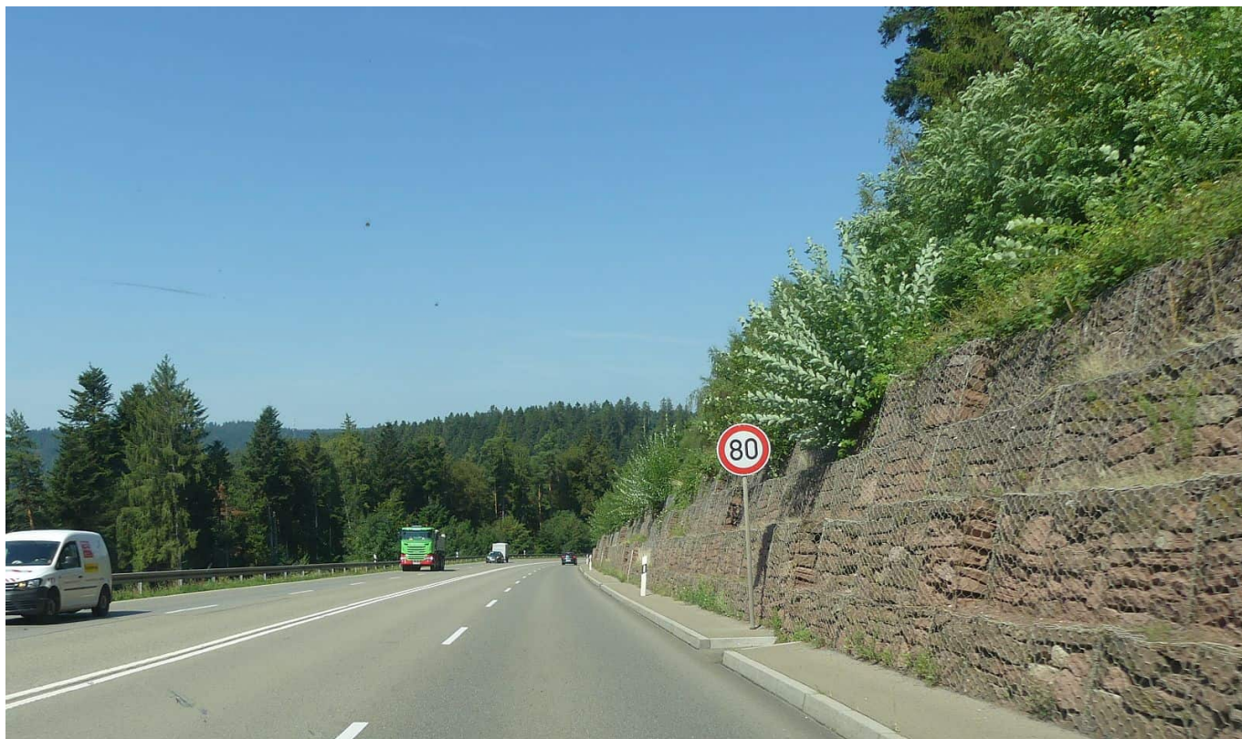
Gabionen am Hang machen Sorge. Foto: him
